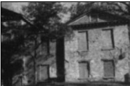
Holt House, National Zoological Park, Adams Mill Road, NW Credit: Wanda Bubriski
